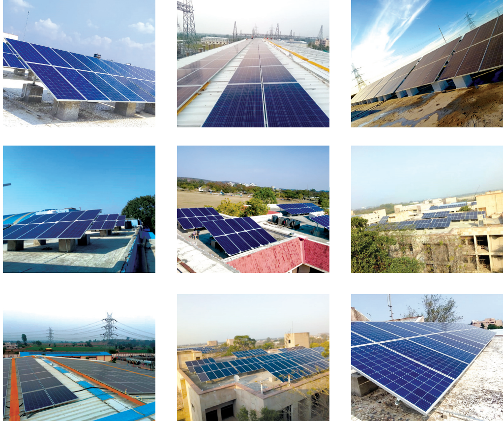
The RESCO 1 and 2 installations
